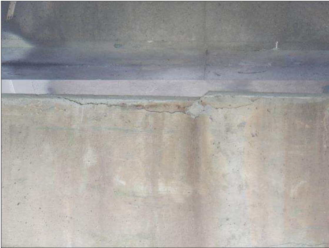
Bent 1 Cap 1: 3 FEET X UP TO 1/8 INCHES HORIZONTAL CRACK ON SPAN 1 FACE UNDER BAY 1
