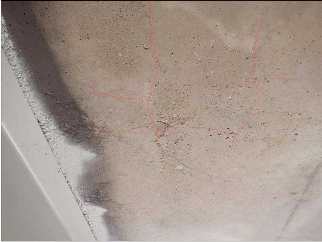
Span 4 Deck: 400 SQUARE FEET OF MAP CRACKING UP TO 1/32 INCHES AT RANDOM THROUGHOUT UNDERSIDE OF DECK
