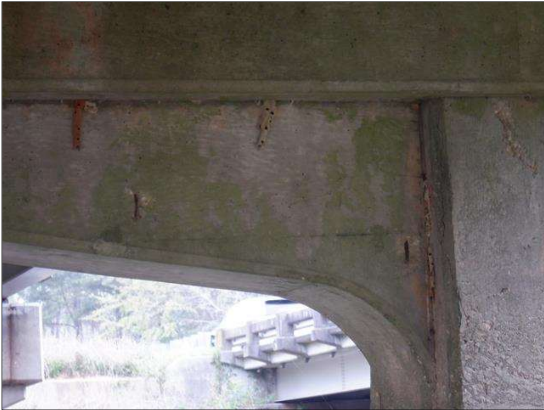
Bent 1 Cap 1: (2) UP TO 3 INCHES X 3 INCHES X 1 INCHES DEEP SPALLS WITH EXPOSED REBAR ON CORBEL OF SPAN 1 FACE
