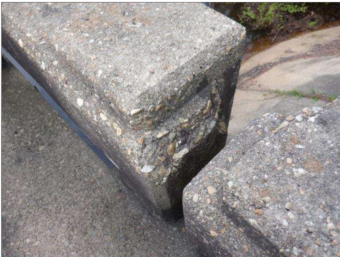
Span 4 Left Concrete Rail: 1 INCHES X 4 INCHES X 2 INCHES DEEP SPALL ON CONCRETE POST 6
