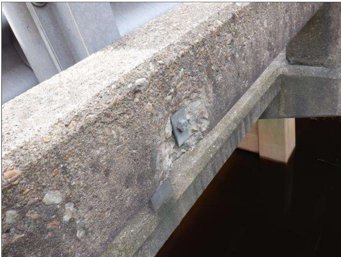
Span 2 Left Concrete Rail: (4) UP TO 9 INCHES X 6 INCHES X 1 INCHES DEEP SPALLS IN OUTSIDE FACE OF CONCRETE RAIL, AT RANDOM
