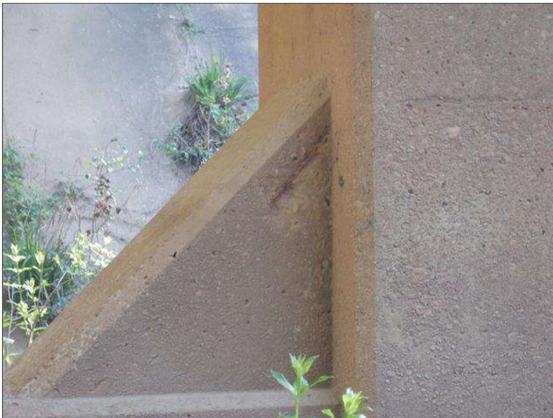
Bent 3 Pile 2: 8 INCHES X 4 INCHES X UP TO 1/2 INCHES SPALL WITH EXPOSED REINFORCING ON SPAN 3 FACE OF CORBEL UNDER STRUT.
