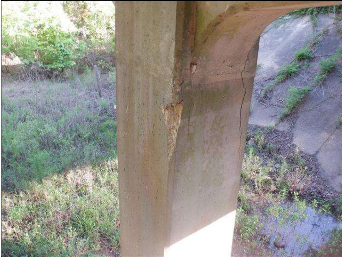
Bent 3 Pile 1: 14 INCHES X UP TO 6 INCHES X 2 INCHES SPALL WITH ADJACENT 1 FEET DIAMETER DELAMINATION ON SOUTHEAST CORNER, 2 FEET FROM BOTTOM OF CAP
