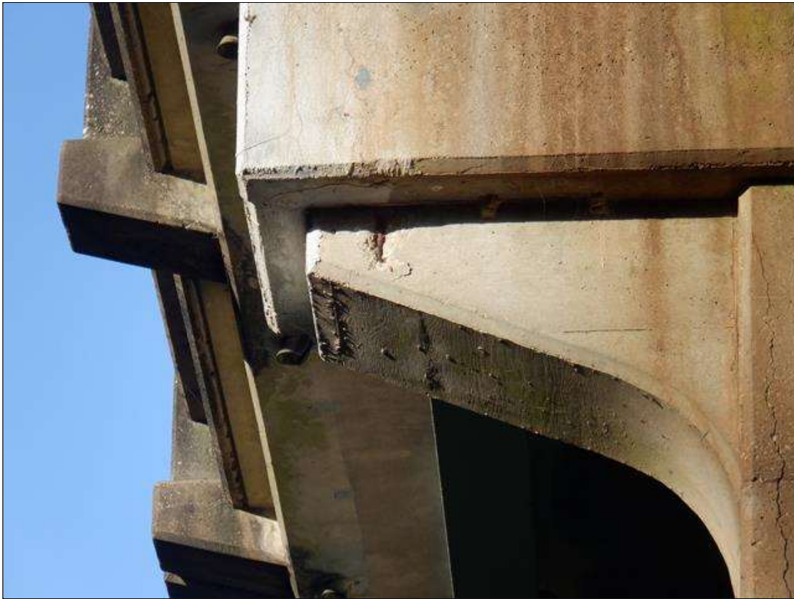
Bent 1 Pile 2: 6 INCHES X 8 INCHES X UP TO 1/2 INCHES SPALL WITH EXPOSED REINFORCING IN NORTH FACE OF CORBEL, UNDER BEAM 4.
