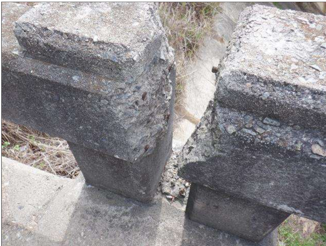
Span 4 Right Concrete Rail: 2 INCHES X 8 INCHES X 10 INCHES DEEP SPALL WITH EXPOSED REBAR ON CONCRETE POSTS 6 AND 7
