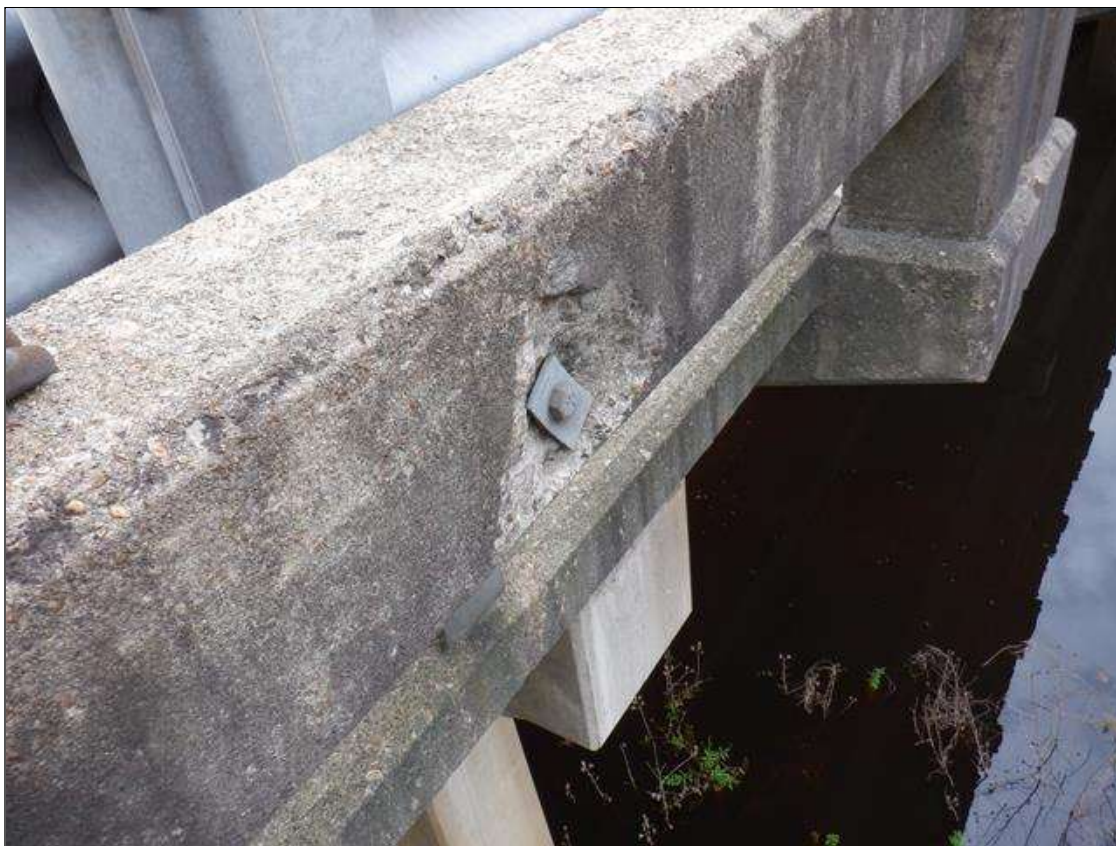
Span 4 Left Concrete Rail: (4) UP TO 10 INCHES X 9 INCHES X 1 INCHES DEEP SPALLS IN OUTSIDE FACE OF CONCRETE RAIL, AT RANDOM
