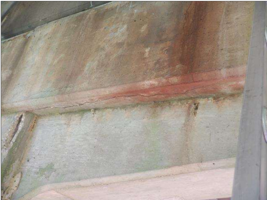
Bent 1 Cap 1: 2- UP TO 6 FEET X 1 INCHES LONGITUDINAL CRACKS WITH ADJACENT 6 FEET X 5 INCHES X 4 INCHES DELAMINATION IN BOTTOM OF SOUTH FACE UNDER BEAM 2.
