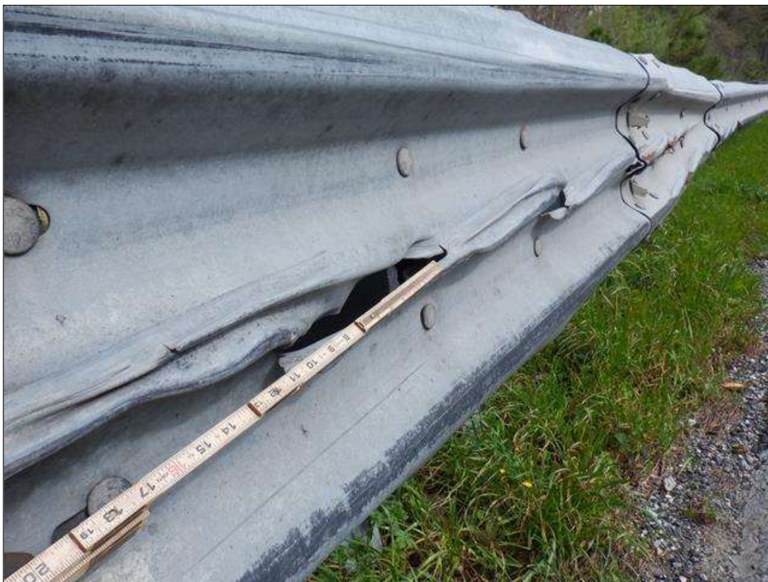
General Comments and Misc. Items: (PAR) 20 FEET OF IMPACT DAMAGE WITH 12- UP TO 10 INCHES X 1.5 INCHES GOUGES IN NORTHWEST GUARDRAIL, 15 FEET FROM END BENT 2.
