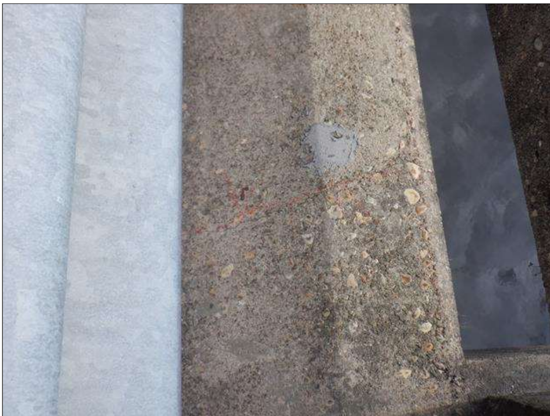
Span 3 Right Concrete Rail: (5) UP TO 1/64 INCHES VERTICAL AND TRANSVERSE CRACKS ON CONCRETE RAIL AND CURB, AT RANDOM
