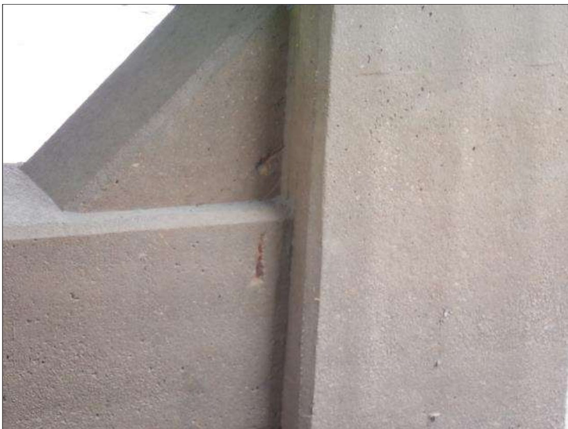
Bent 1 Pile 2: (2) UP TO 3 INCHES X 2 INCHES X 1/2 INCHES DEEP SPALLS WITH EXPOSED REBAR ON CORBEL AND STRUT ON SPAN 1 FACE
