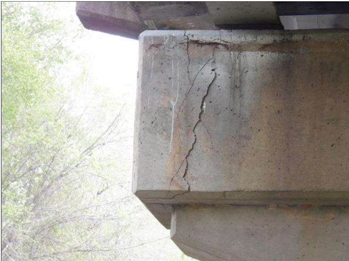
Bent 1 Cap 1: 12 INCHES X 24 INCHES AREA OF DELAMINATION WITH UP TO 1/8 INCHES VERTICAL AND DIAGONAL CRACKS ON SPAN 1 FACE AT WEST END
