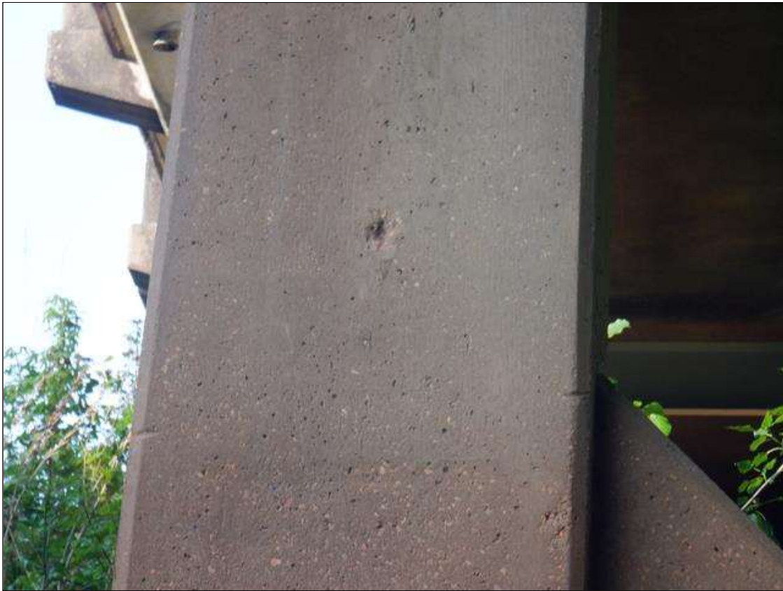
Bent 1 Pile 2: 6 INCHES DIAMETER X UP TO 1/2 INCHES SPALL WITH EXPOSED REINFORCING IN NORTH FACE, 4 FEET FROM TOP OF STRUT.
