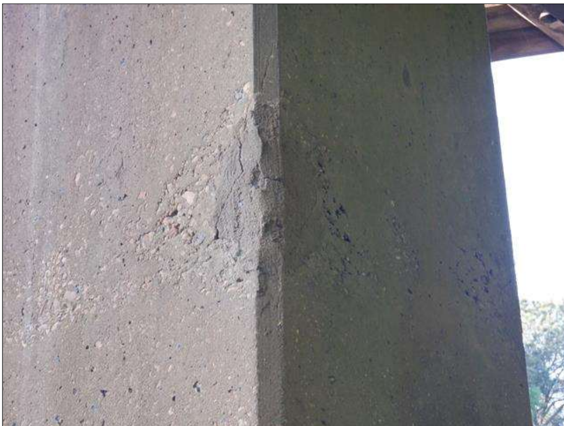
Bent 2 Pile 2: 12 INCHES X 8 INCHES X 4 INCHES CRACKED PATCHED AREA WITH UP TO 1/16 INCHES CRACKING ON NORTHWEST CORNE, 7 FEET FROM BOTTOM OF CAP.
