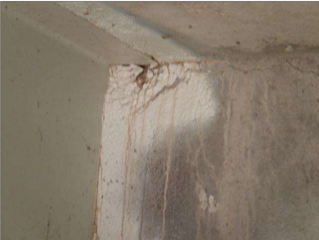
End Bent 2 Abutment: 10 INCHES X UP TO 6 INCHES X 3/4 INCHES SPALL IN BAY 1, ADJACENT TO TOP FLANGE OF BEAM 1.
