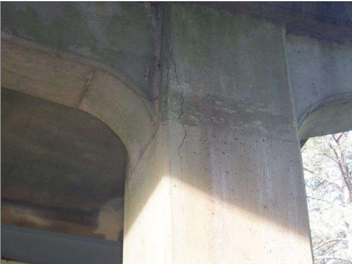
Bent 1 Pile 1: 6 FEET X UP TO 1/8 INCHES VERTICAL CRACK IN NORTHEAST CORNER, 1 FEET FROM BOTTOM OF CAP.
