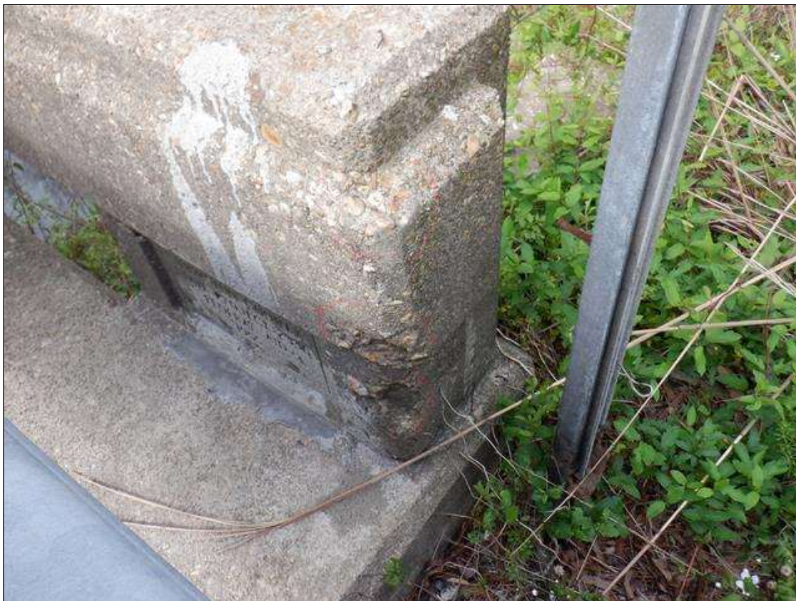
Span 4 Left Concrete Rail: (3) UP TO 3 INCHES X 5 INCHES X 1 INCHES DEEP SPALLS ON END POST
