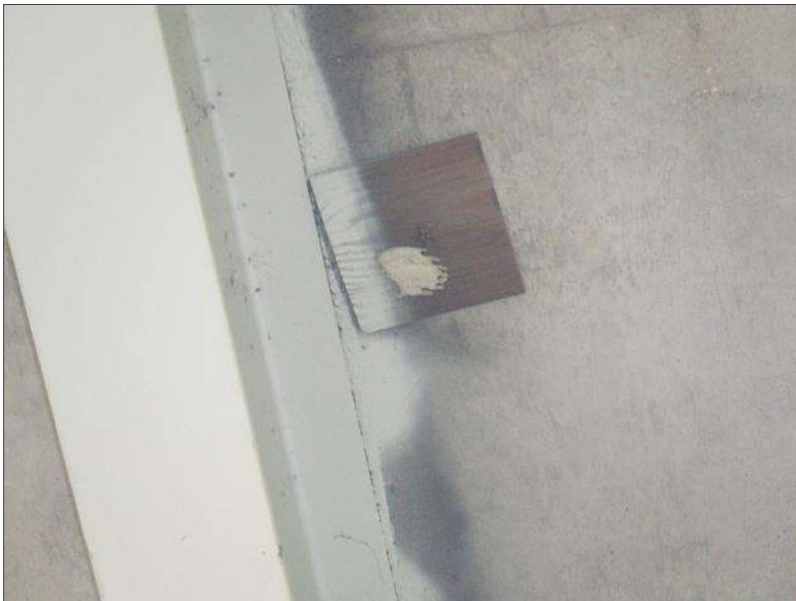
Span 3 Deck: 1 FEET X 1 FEET TIMBER PATCH IN BAY 2, 8 FEET FROM BENT 2, ADJACCENT TO BEAM 3.
