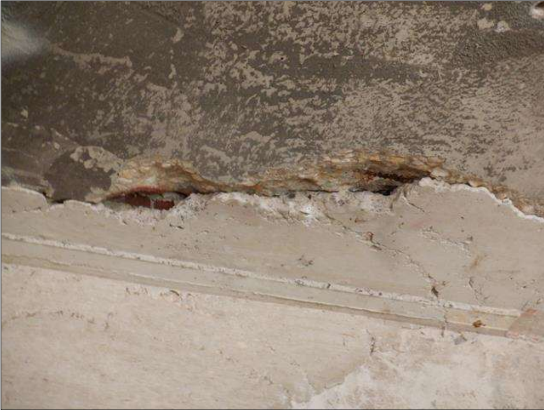
Span 4 Deck: 17 INCHES X 4 INCHES X 2 INCHES DEEP SPALL WITH EXPOSED REINFORCING AND ADJACENT 5 FEET X UP TO 18 INCHES PATCHED AREA IN UNDERSIDE OF DECK IN BAY 2 AT END BENT 2
