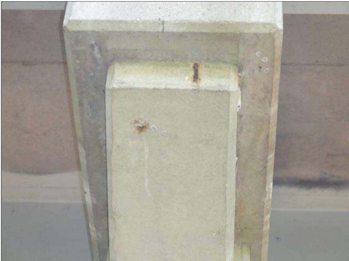
Bent 3 Pile 1: (2) UP TO 3 INCHES X 6 INCHES X 1 INCHES DEEP SPALLS WITH EXPOSED REBAR ON WEST AND BOTTOM FACE OF CORBEL.
