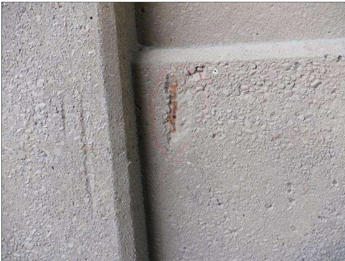
Bent 2 Pile 2: 2 INCHES X UP TO 6 INCHES X 1/2 INCHES SPALL WITH EXPOSED REBAR ON NORTH FACE OF STRUT, NEAR PILE 2.
