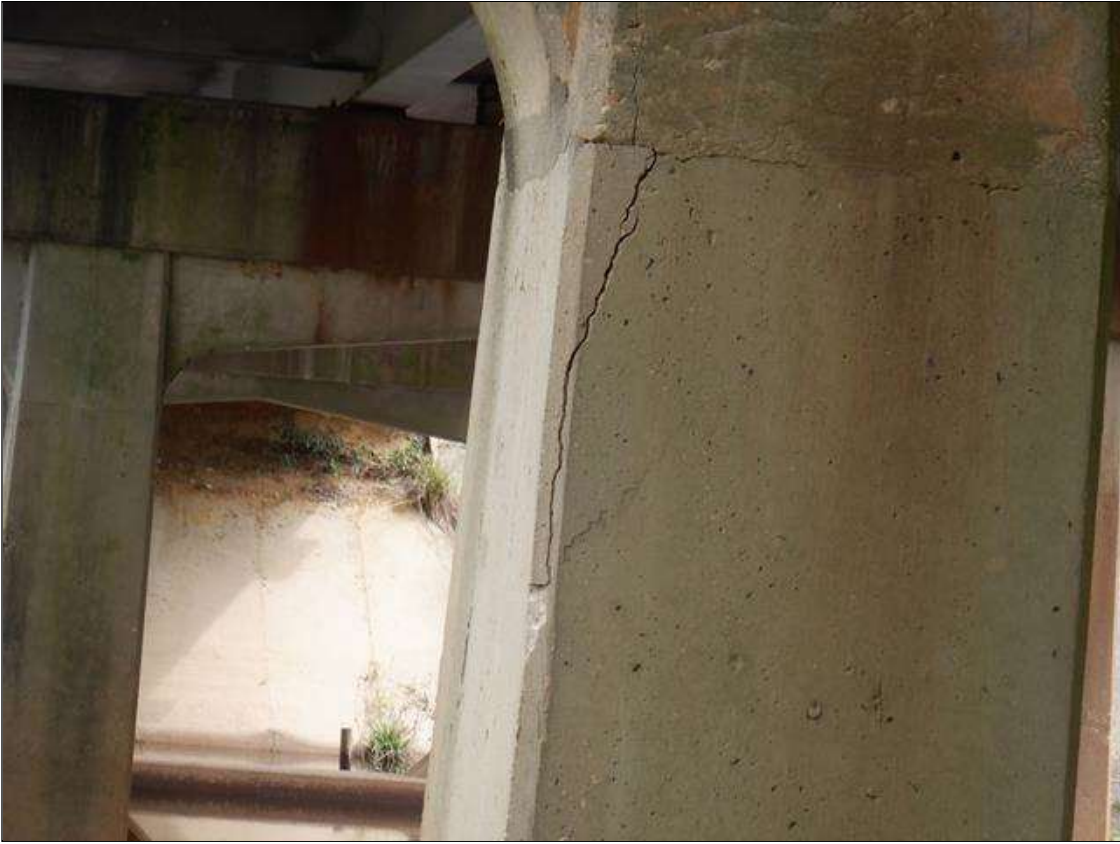
Bent 1 Pile 1: 42 INCHES X UP TO 1/4 INCHES VERTICAL CRACK WITH ADJACENT 4 FEET X UP TO 5 INCHES X 3 INCHES DELAMINATION ON SPAN 1 FACE
