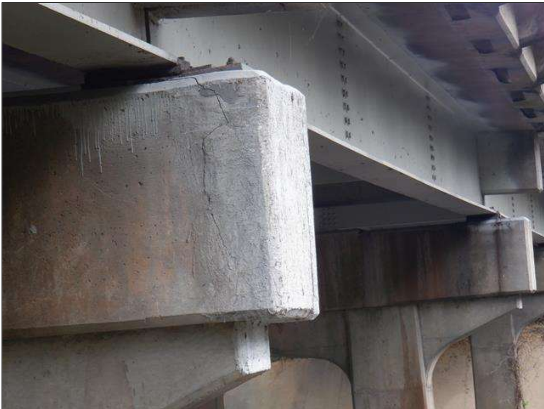
Bent 1 Cap 1: FULL HEIGHT X FULL WIDTH CRACKED PATCHED AREA UP TO 1/16 INCHES ON EAST END OF CAP, EXTENDING 9 INCHES ONTO SOUTH FACE.
